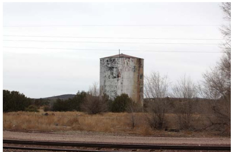
Abandoned Tank at Ash Fork
