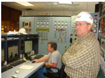
The control room at the plant. Guy on right is the General Manager of the plant and our guide.
