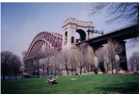
Hell Gate Bridge (above ) crosses the Hell Gate portion of the East River into Astoria Park, Astoria, Queens County, NY. Note the hallmark steel arch, the massive towers with tall portals, the piers supporting the viaduct and the catenary towers (Guys -- Forget the sunbathers -- this is a family newsletter). The arch
