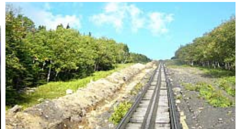
Above pictures show the work being done to put in the snow making equipment.
